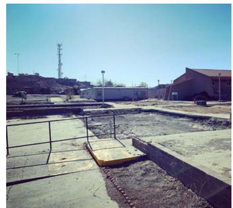
Modular buildings were removed during phase I of NTU's 30,000 sq. ft. classroom building. COVID halted construction.
