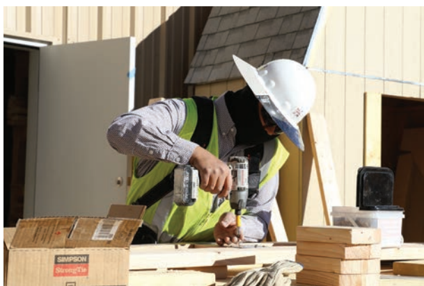
Construction Technology instructor Tom Bebo provides guidance to students as part of the bathroom addition project with Navajo Solutions. Navajo Solutions was created to provide hands on training in professional trades leading to permanent job placement.
